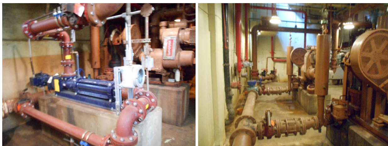
FIGURE 3-31 DIGESTED SLUDGE TRANSFER PUMPS
