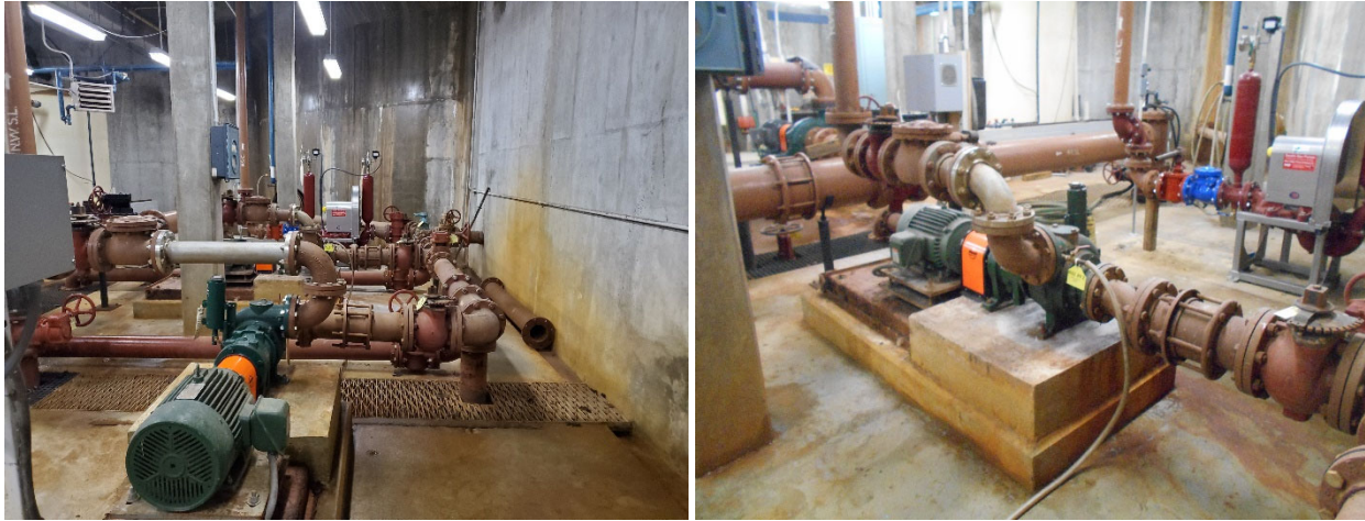
FIGURE 3-19 NITRIFICATION-WASTE ACTIVATED SLUDGE PUMPS
