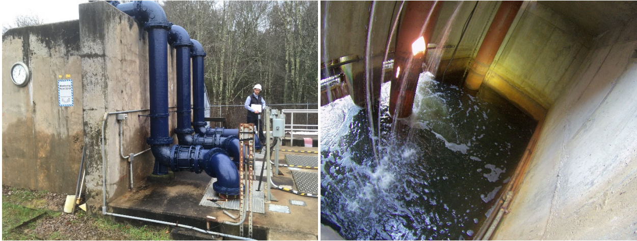
FIGURE 3-21 EFFLUENT PUMP STATION
