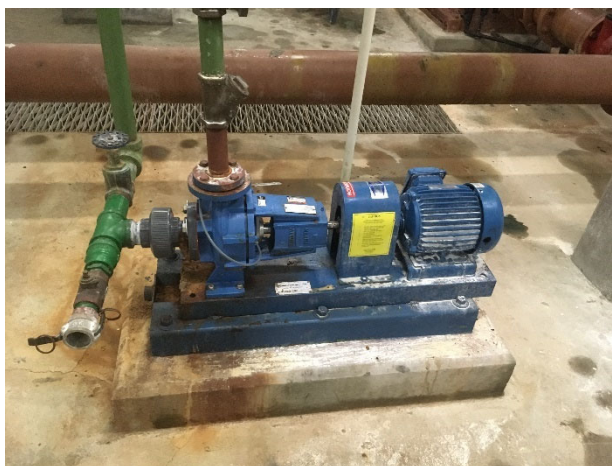
FIGURE 3-36 PLANT WATER PUMPS
