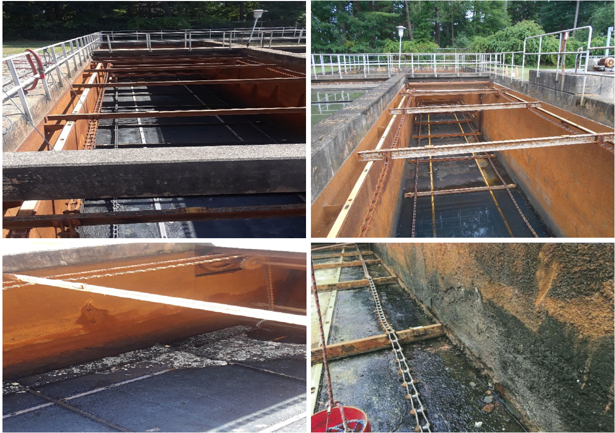
FIGURE 3-11 LARGE PRIMARY SETTLING TANKS
