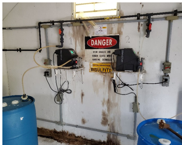
FIGURE 3 26 SODIUM BISULFITE PUMPS
